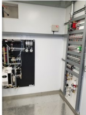
Inside a CEMS Shelter
