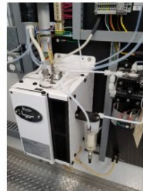
Extractive Conditioning System
