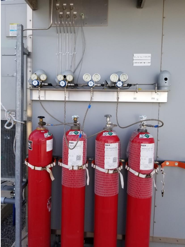
Cylinders of EPA Certified Gases
