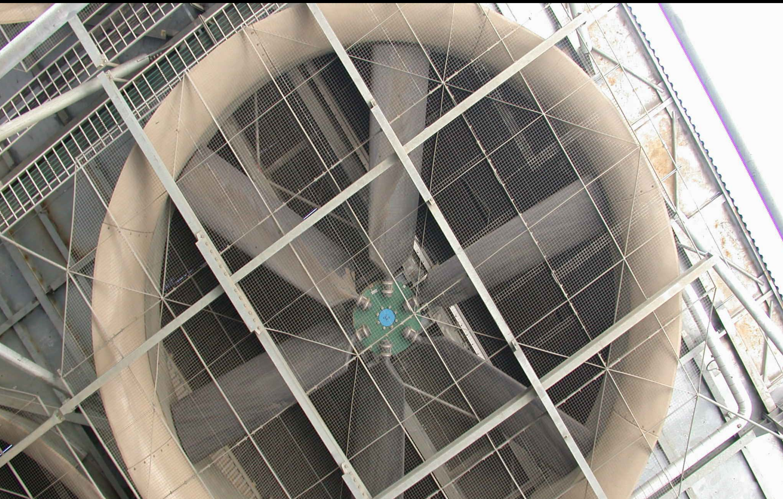
Dry Air-Cooled Condenser Fans
