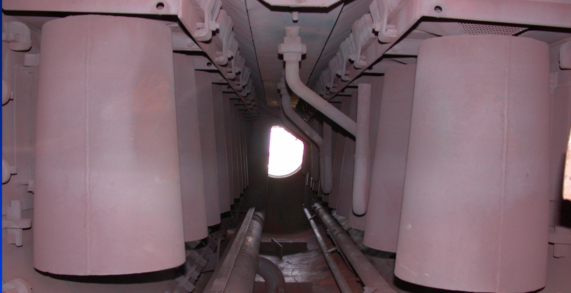
Steam Drum w/Cyclone & Chevron Separators
