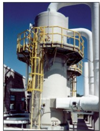
Packed Towers are primarily used for gas absorption.
