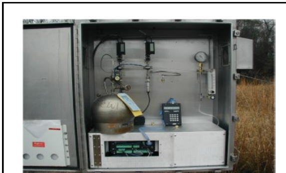
Example of Compendium Method TO-15 at Typical Ambient Monitoring Site.
