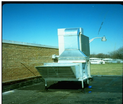
Smaller 1500 CFM Baghouse with carbon after filters on Paint mixing Operation
