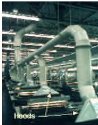
Figure 3-12. Stationary hood in an industrial process.
