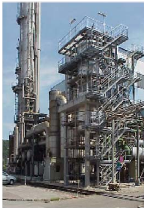
Figure 10-16. Uhde EnviNO x ® reactor in Linz, Austria. Source: ICAC, 2009.
