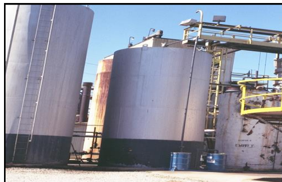
Non-Regenerable Carbon Adsorption Drums controlling mercaptan odors from re-refined crankcase oil product 4 - 106
