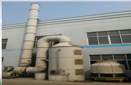
Counter-current Packed Tower at a Plating Operation
