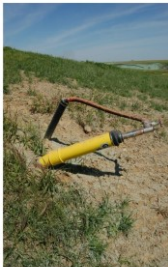
Photo 2. Storage Use Collection line (Source: DMR Staff, 2012).
