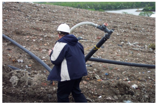
Landfill Vertical Gas Extraction Well
