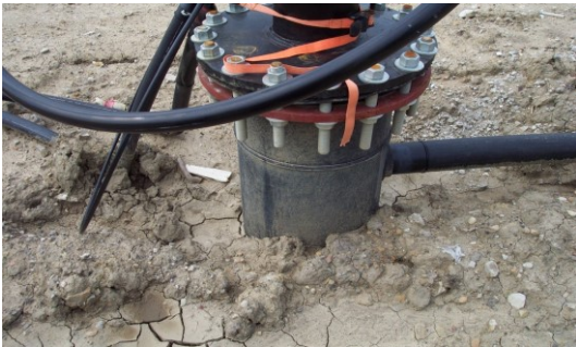
Leachate Extraction Well Riser
