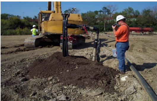
Combination Extraction Well at Landfill
