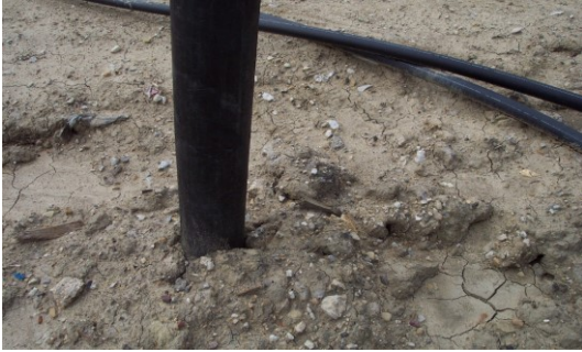
Vertical Landfill Gas Extraction Well
