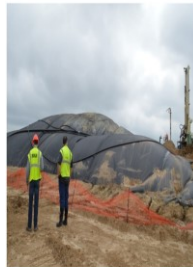
Photo 4. Excessive Landfill Gas and Inflated FNL, May 2013 (Source: DMR Staff, 2013).
