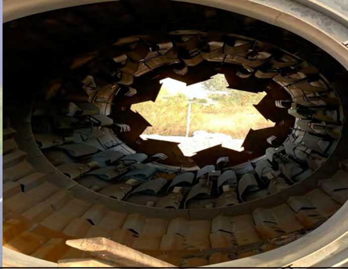
Inside View of Double Drum Dryer Section
