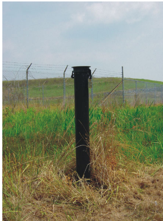
Perimeter Gas Monitoring Probe
