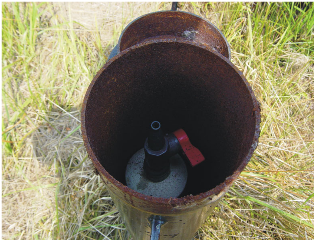
Encased Valve to a Perimeter Gas Monitoring Probe
