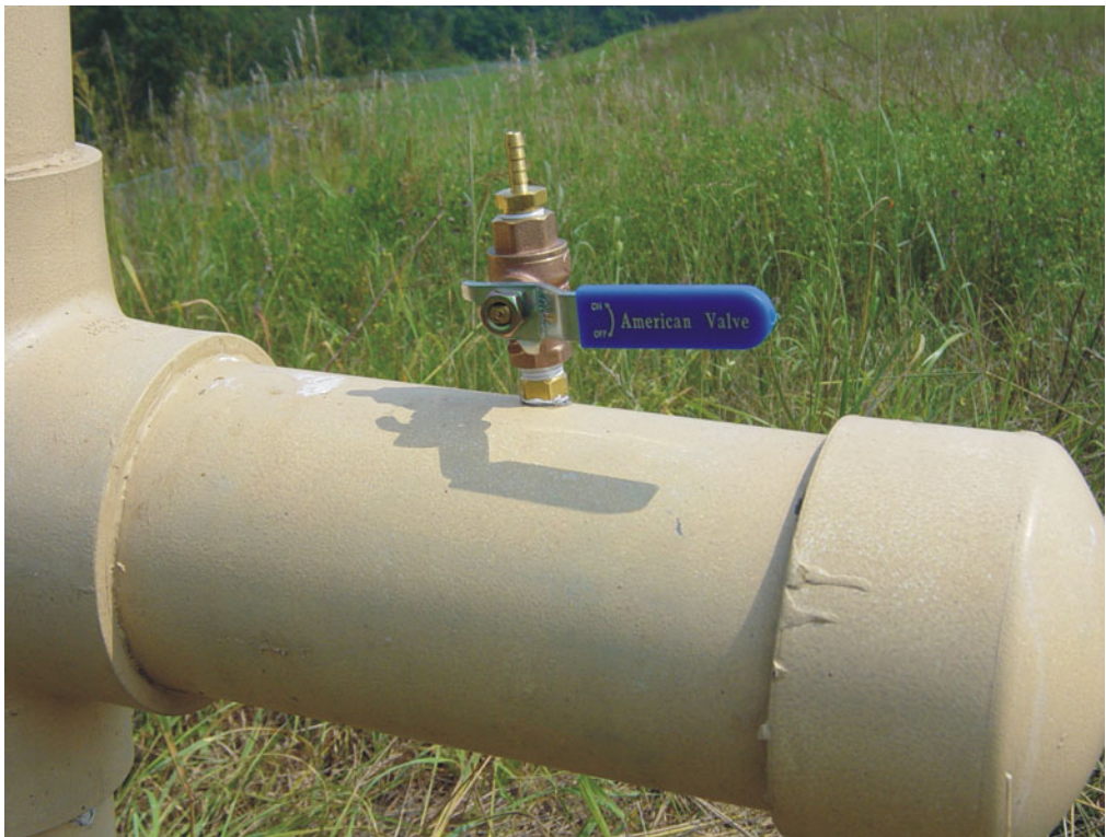
Sampling Valve Installed on a Passive Vent
